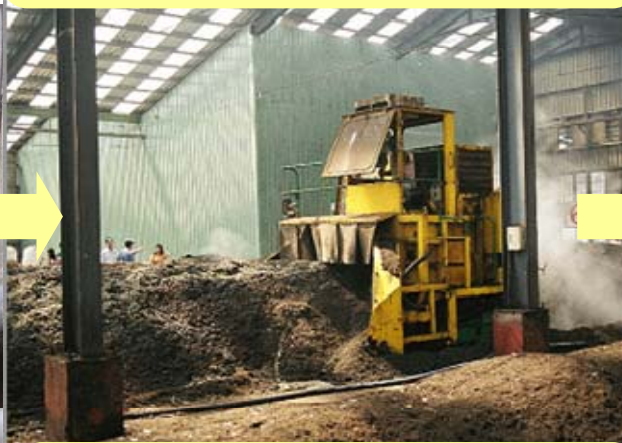
5. 堆肥場 Composting Treatment
